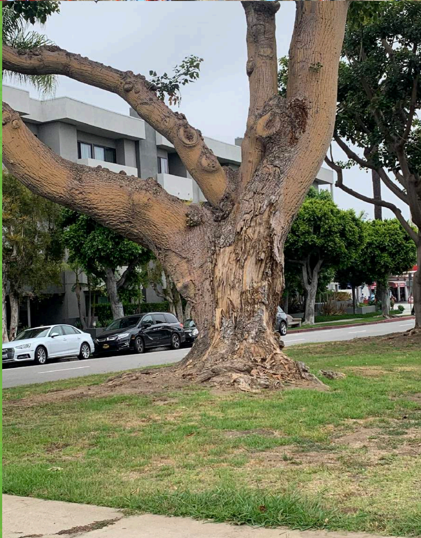
City of LA Coral tree - with decay at the base
